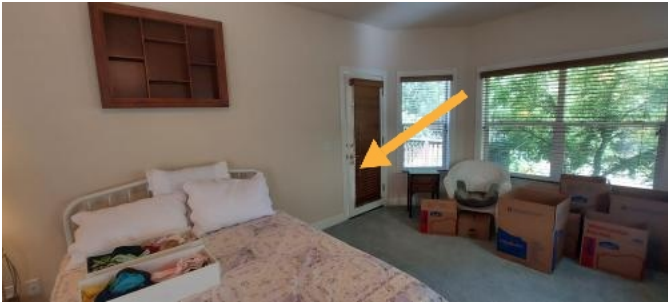
This door sticks at the door frame here.
