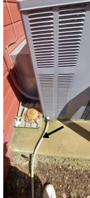
Garden hose ysed as a drain.
