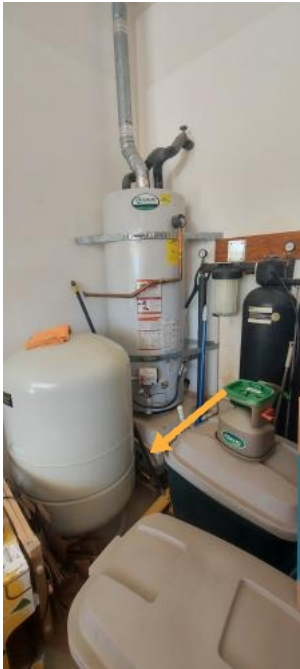
Water main valve location
